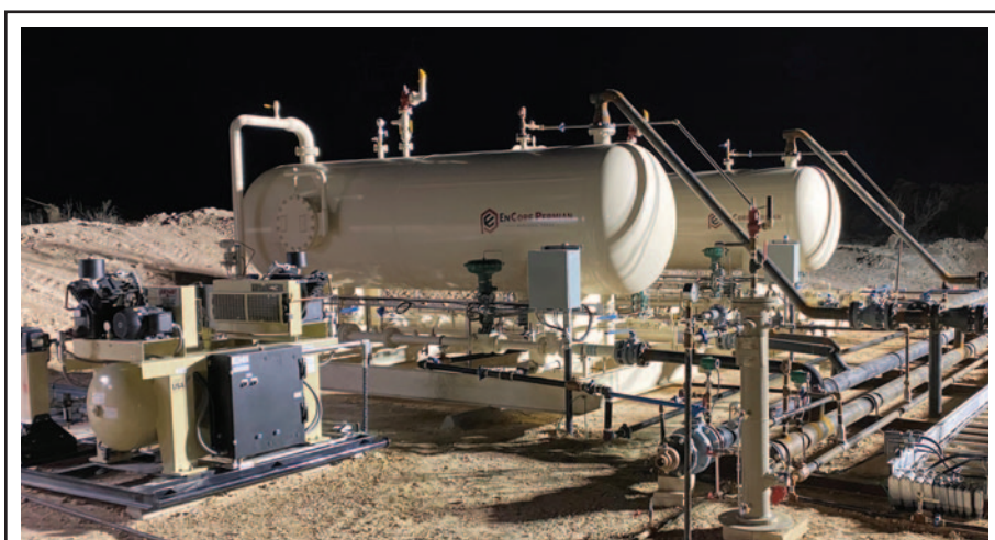
Automated air compressor skids ensure that clean and dry instrument air is available around the clock with built-in redundancy and fail-safe systems to operate all key separator, heater treater, freshwater knockout and other equipment functions. The skids integrate an industrial-grade air compressor with aftercoolers, air tanks, low-maintenance dryers and electric automation and smart logic.
