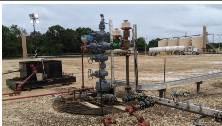
Automated wellhead chokes regulate flow volumes to continue production while staying within flaring limits, and also can dramatically reduce proppant flowback by maintaining consistent backpressure to eliminate “burping” events that send sand up the wellbore. Shown here is a well with both an automated wellhead emergency shutdown valve and automated wellhead chokes.
